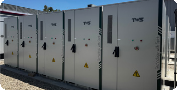
3.75 MW/ 7.45 MWh Manufacturing, US
