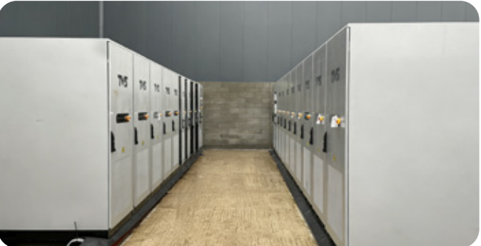
2.5 MW/ 5.24 MWh Food Processing, Belgium
