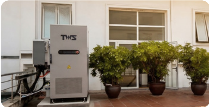
125 kW / 262 kWh Municipal Building, Vietnam
