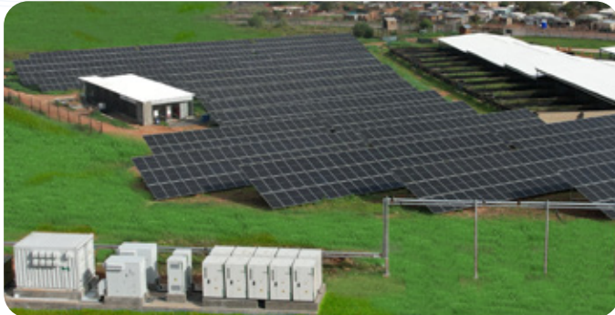
4.7 MW/ 5.9 MWh Agriculture & PV, South Africa
