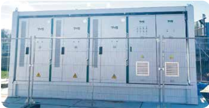
500 kW/ 978 kWh Municipal Sewage Treatment, Netherlands
