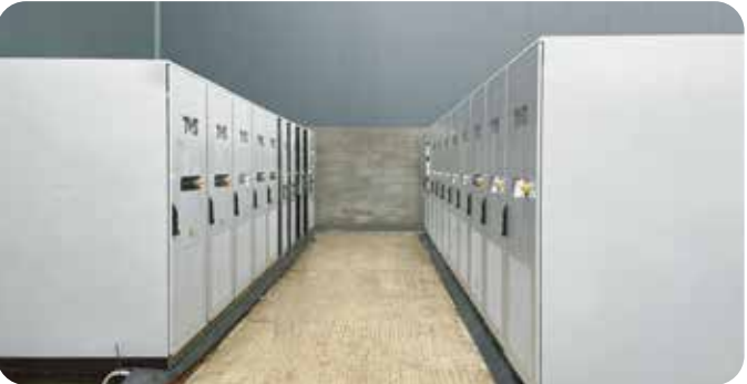
2.5 MW/ 5.24 MWh Food Processing, Belgium
