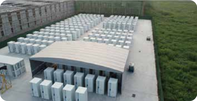
225 MW/ 450 MWh Steel Production, China
