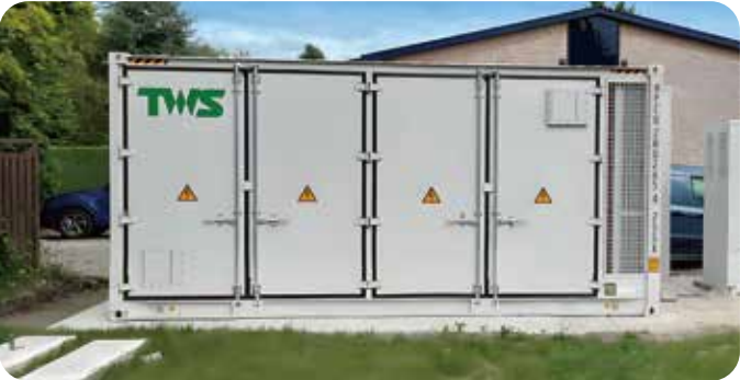
1.72 MW/ 5 MWh Horticulture, Netherlands
