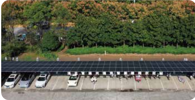
1.2 MWh Intelligent Microgrid, China
