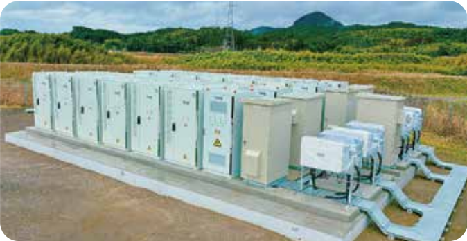
2MW / 6.7 MWh Utility, Japan
