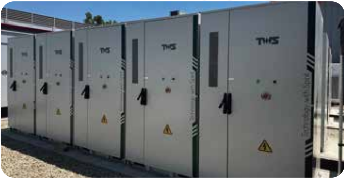
3.75 MW/ 7.45 MWh Manufacturing, US
