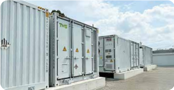
2 MW/ 8 MWh Utility, Japan
